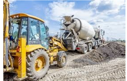
▲ Large moving vehicles are always a major hazard on site
