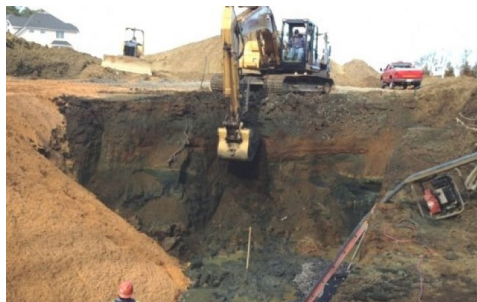
▲ A shocking example of an unguarded deep excavation
